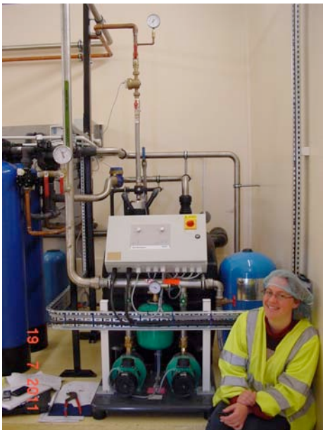
The Rainwater control unit in situ.
