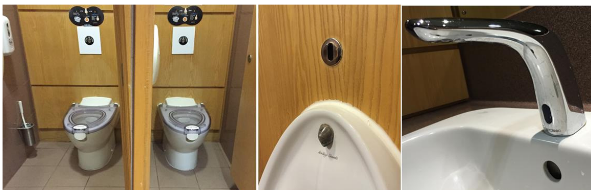
Figure one: Photos of the three water efficient devices fitted.
