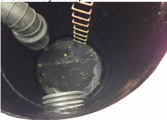
3. Secondary silt trap
